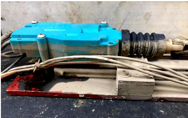
T33 Actuator; Note the high water line & mud!
