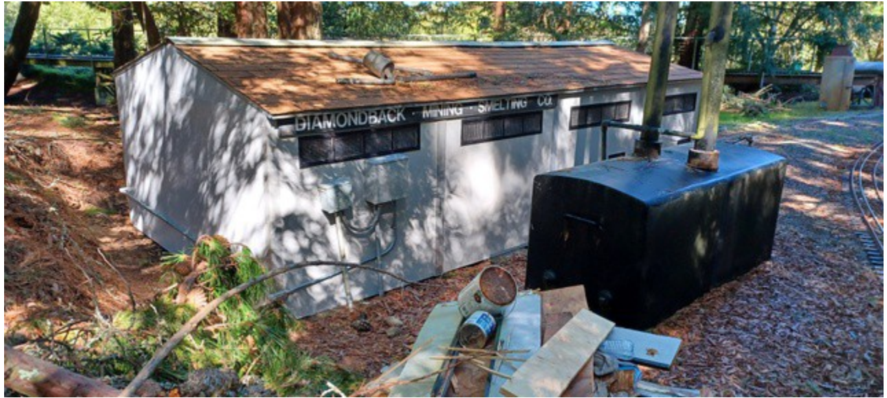
Diamondback Mine Refurbishment Completed! More information can be found in this issue.
